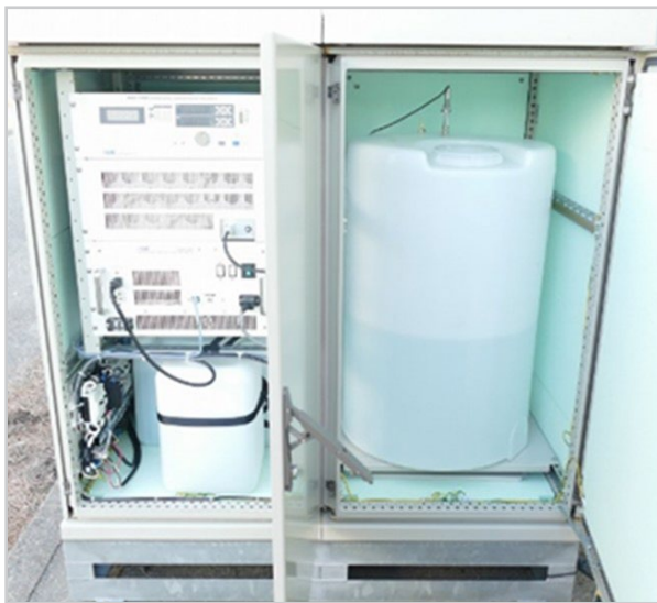
Inside the DMFC cabinet
