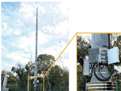
Private BWA base station with 30-meter antenna mast and wireless station terminal at the Chiba Plant
