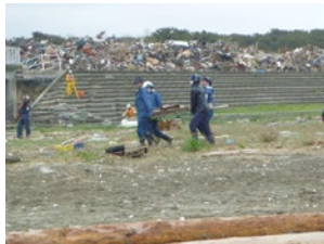
Ishinomaki City, May 2011. Work to clear flotsam on the coast began right after the earthquake.
