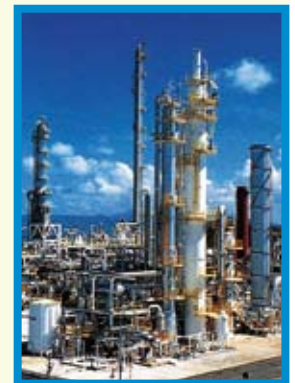
MHI's CO 2 recovery units can capture up to 450 tons of CO 2 per day
