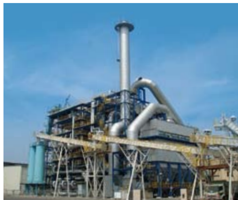
The main facility of the Gonoike biomass power plant
